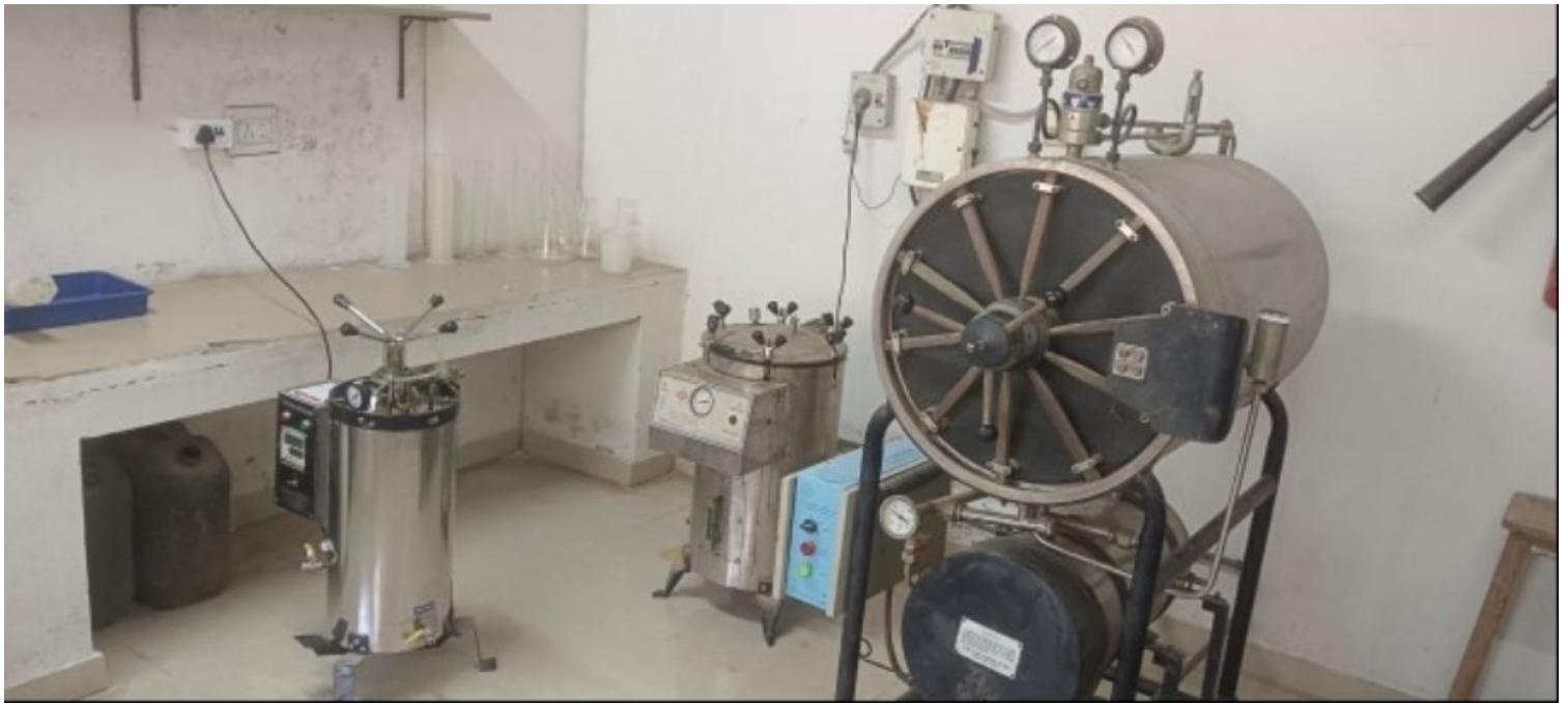
Vertical and Horizontal Autoclaves in Microbiology Preparation Room
